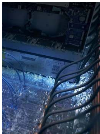
Immersion Cooling Systems
